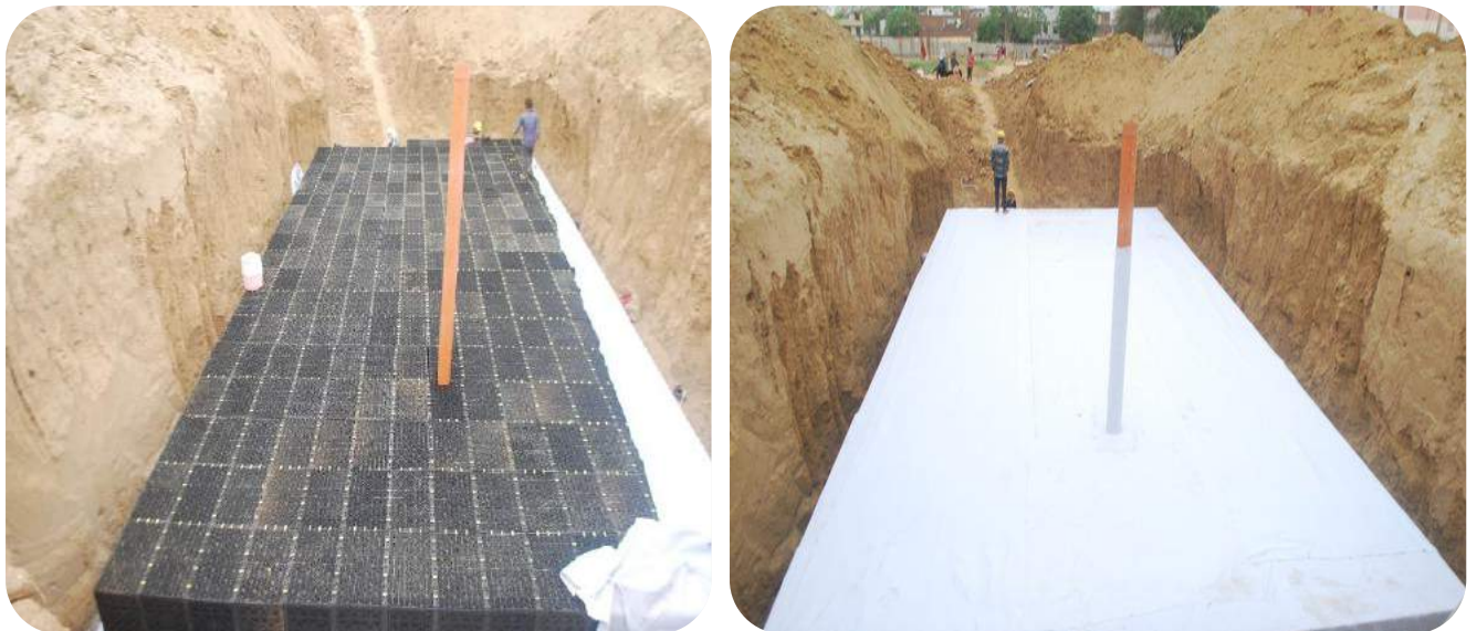
Figure 21: Actual site installations
